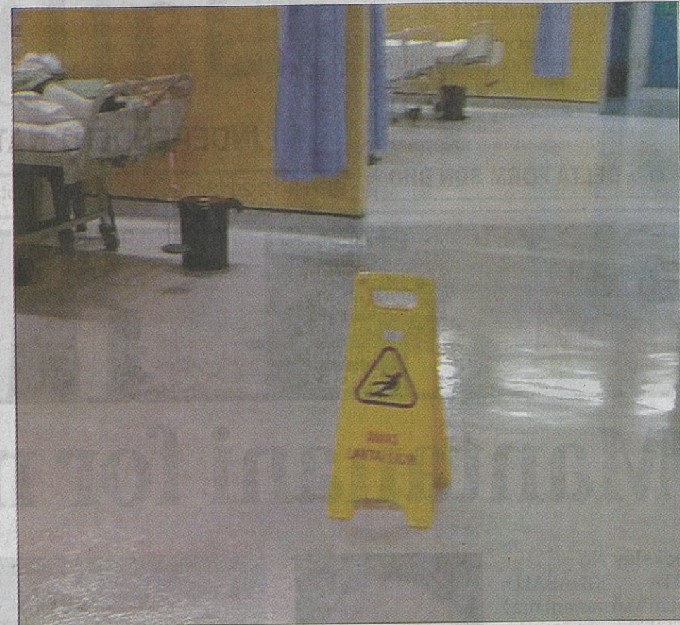
The wet floor due to the leaking hospital roof.
